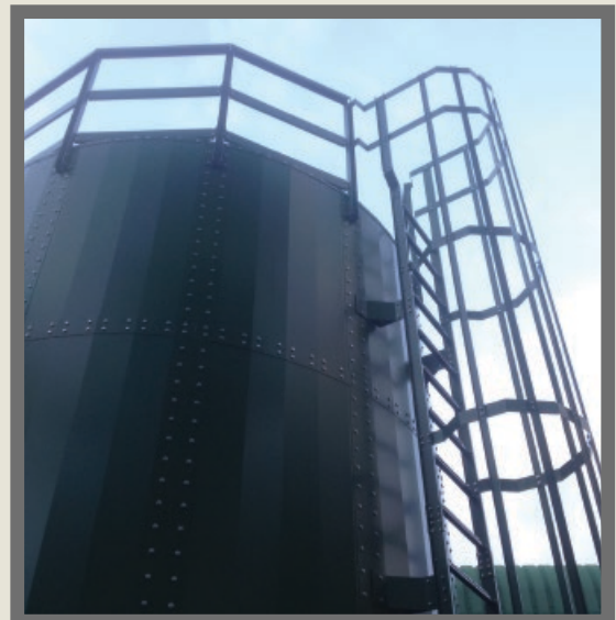
Access Ladder – Including roof access panel.
